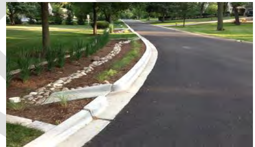
Figure 8. Green Road with Bioswale
