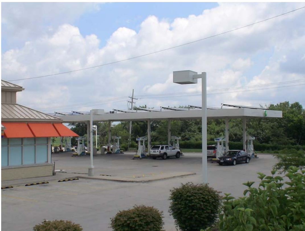
Example of a Building-Mounted Solar Energy System
