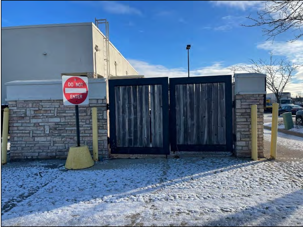
Existing Trash Enclosure Doors To Be Repaired
